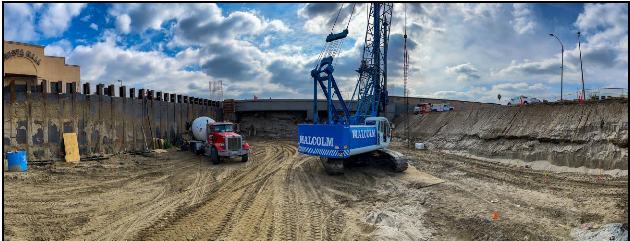
Picture 2: Installing retaining wall foundation system and excavating Durfee Avenue approaching the new railroad bridge.
