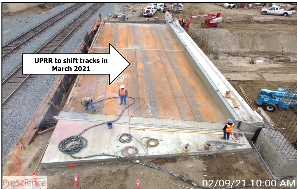
Picture 1: Phase 1 of Rail Bridge nearly complete. Workers are preparing the steel surface for waterproofing. UPRR will then lay their tracks over the completed bridge starting in mid-March 2021.
